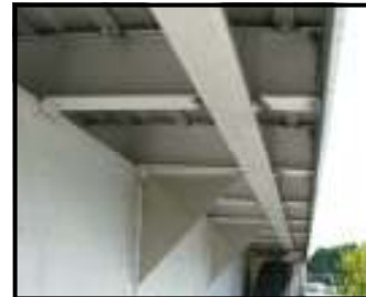
Under deck tie bar
